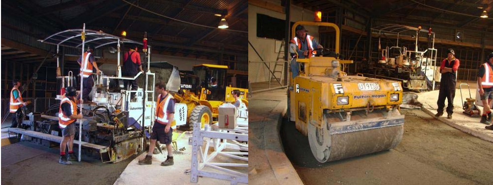
Figure 7 (a) Paver used to spread the basecourse in CAPTIF (b) Compaction of basecourse
