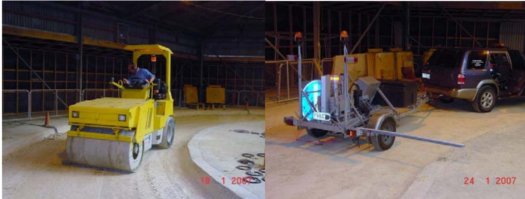
Figure 6: (a) Compaction of subgrade lifts using CAPTIF roller (b) FWD testing on subgrade
