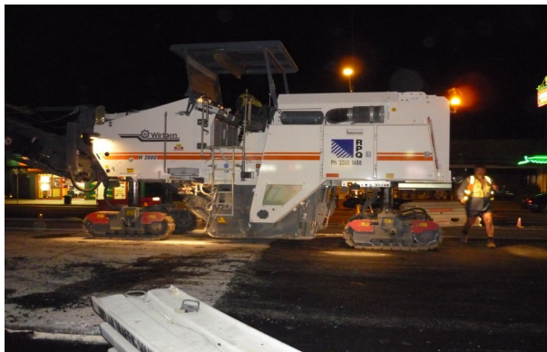
A milling machine removing the top layer of an asphalt pavement on the Gold Coast.
