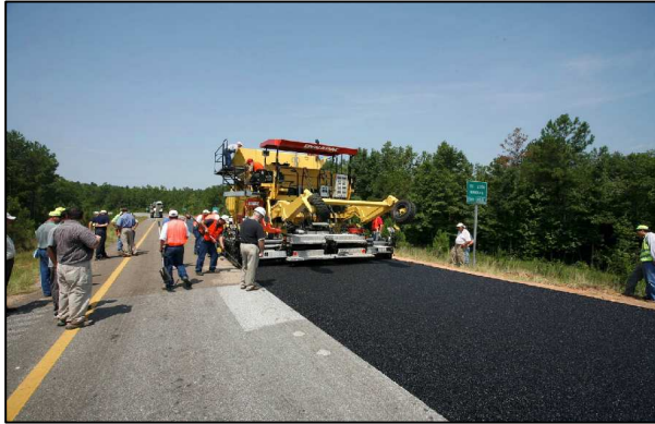
Fig. 8: View of the testing site of NCAT. 24 months of constant loads atop the testing fields. (Photo: NCAT)
