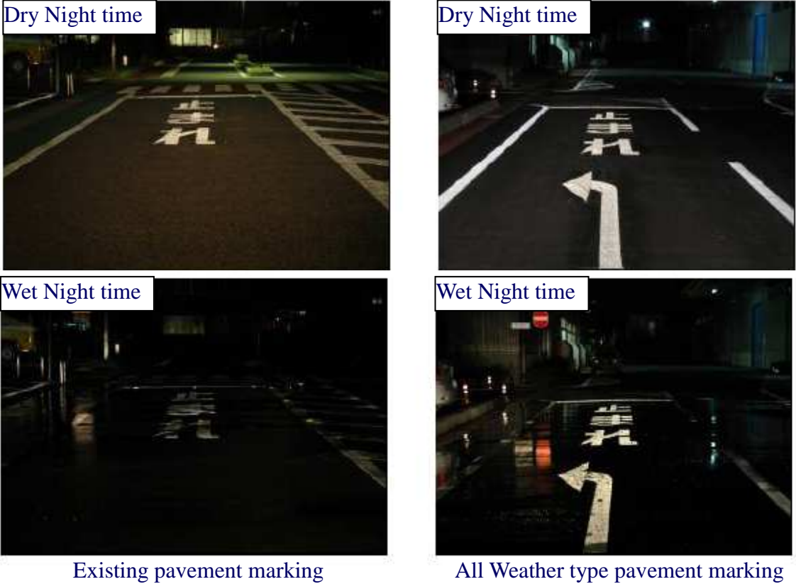
Figure 12: Photo of existing and all weather pavement marking applied on the road
