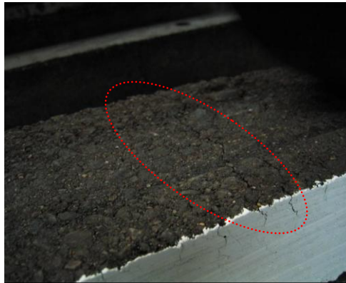
Photo 4: Cracking occurred in mixture surface (Dense-graded mixture used PMA- II).
