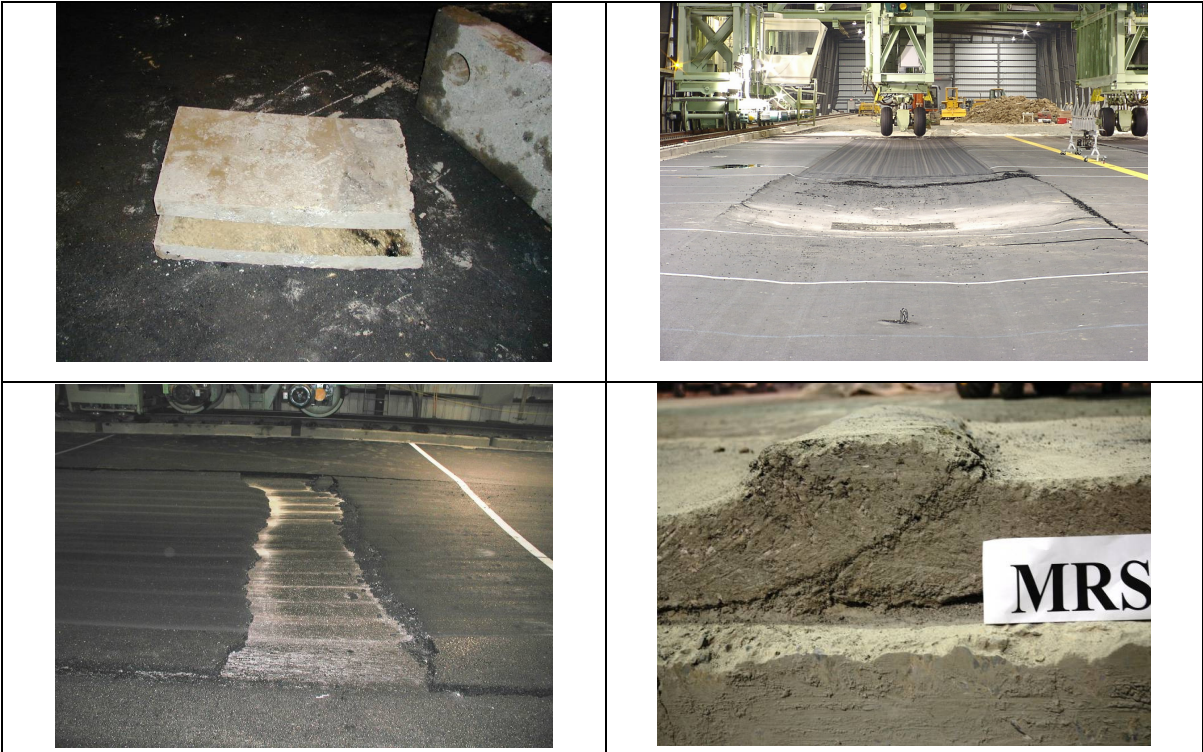
Figure 2: HMA distresses observed during full-scale, accelerated pavement testing at the NAPTF.
