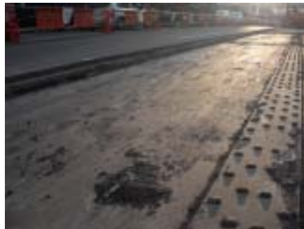
Photo 8: Removal Scene (Insufficient Heating)
