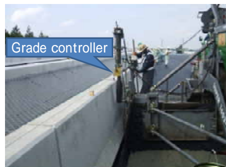
Photograph 1: Establishing a reference line on the top of the railing, and an automatic lift height control system
