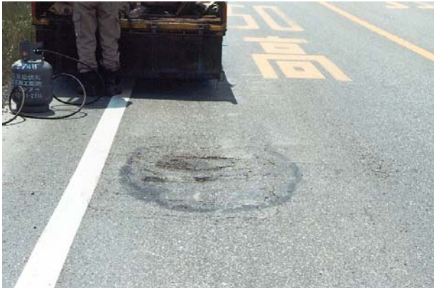
Photograph2: Spot to be repaired, a depression with cracks
