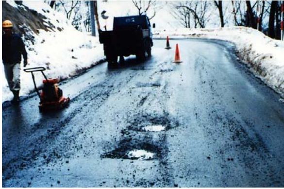
Photograph12: Pot holes to be repaired in snow-melting season
