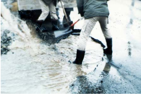
Photograph8: Spot to be repaired, a pot hole with water
