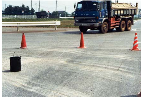
Photograph5: Spot to be repaired, a depression in an intersection
