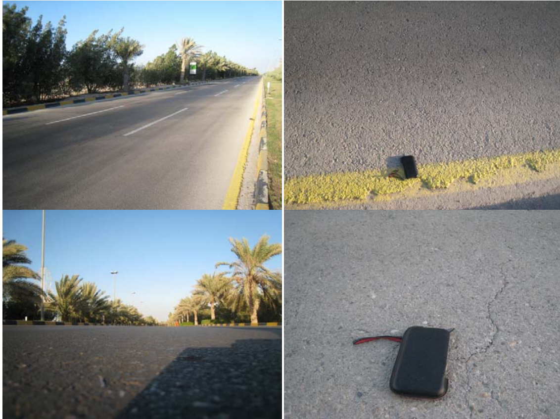
Figure 7: Surface condition of the roads four years after rehabilitation
