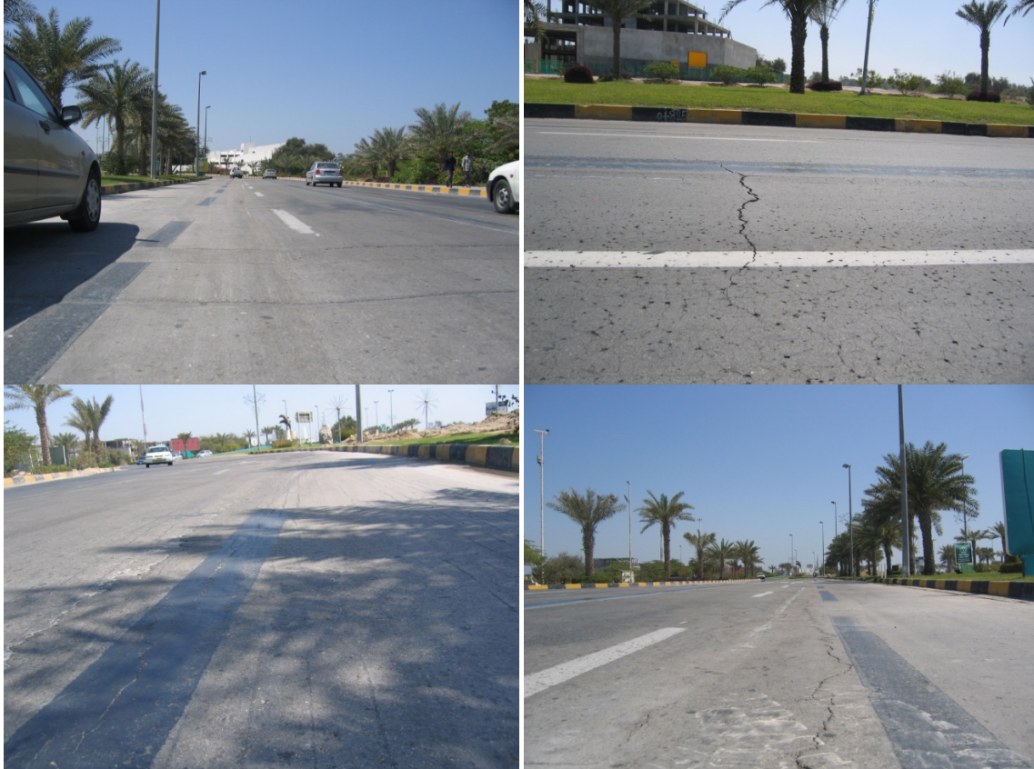
Figure 6: Surface condition of the roads before rehabilitation
