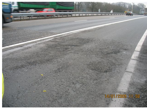
Figure 3: Difference in raveling new/old PA
