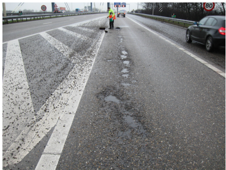
Figure 4: Example of potholes in PA.
