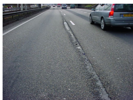
Figure 5: Example of an open longitudinal joint
