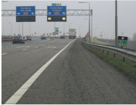
Figure 2: Example of severe raveling
