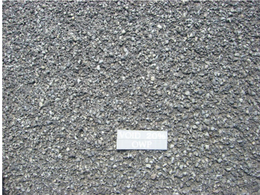
Photograph 2: Porous HMA pavements right after the raveling of aggregate
