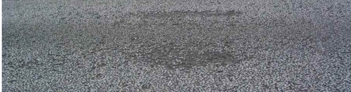
Figure 1: Example of raveling on a HRA surface.
