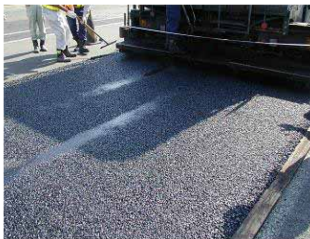
Photo 2: Bitumen's run-off problems
