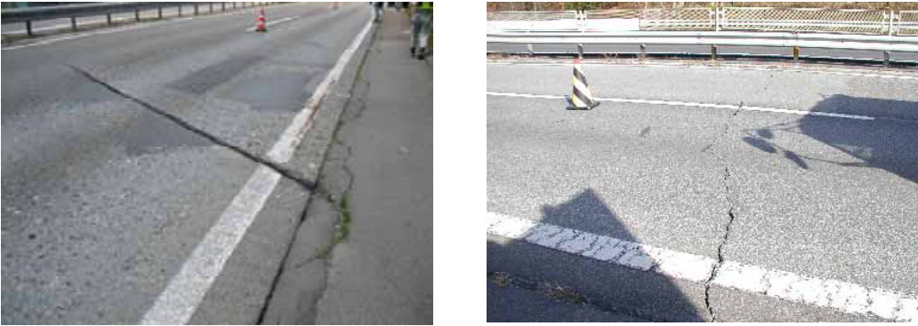
Figure2: Joint faulting (left) and transverse crack (right)
