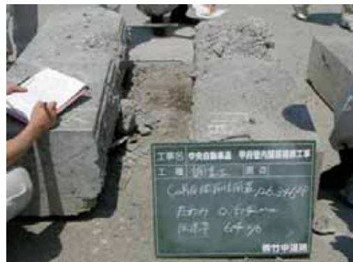
Figure 6: Point with slip bars broken (load transmission 64%)
