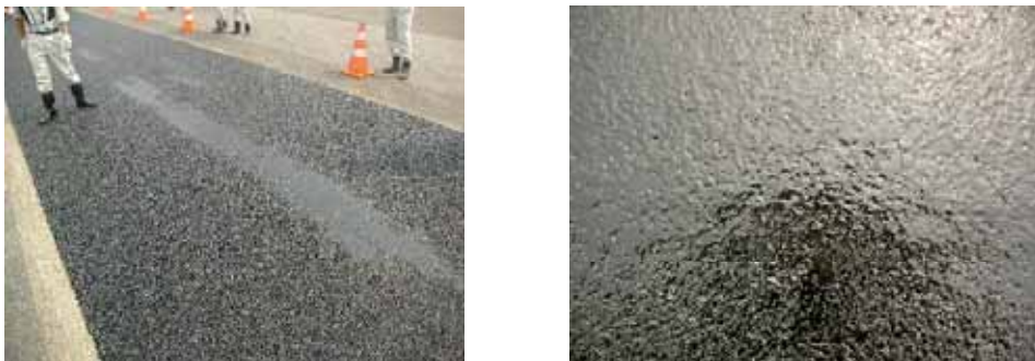
Figure 9: Asphalt run-off problems (Ordinary modified asphalt, SBS 4%)
