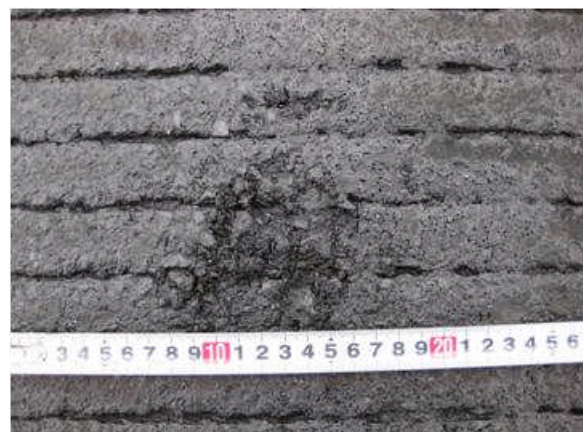
Figure 5: Cutback of the asphalt surface caused by fuel leakage
