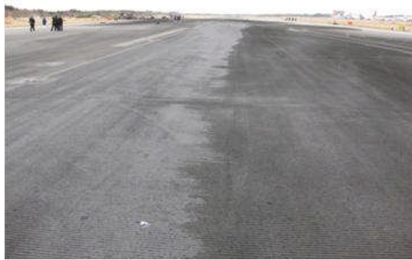
Figure 4: Damaged runway surface
