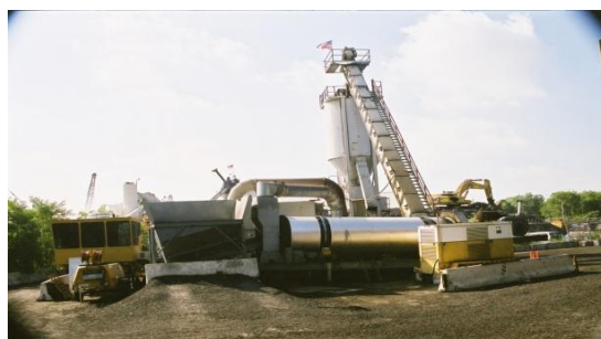
Figure 4: NYCDOT 100% Recycle Pilot Plant
