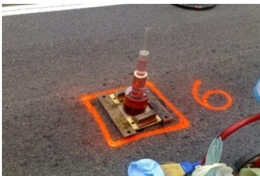
Figure 2: More permeable pavement
