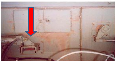
Photo 5: Piston for Gate Opening
